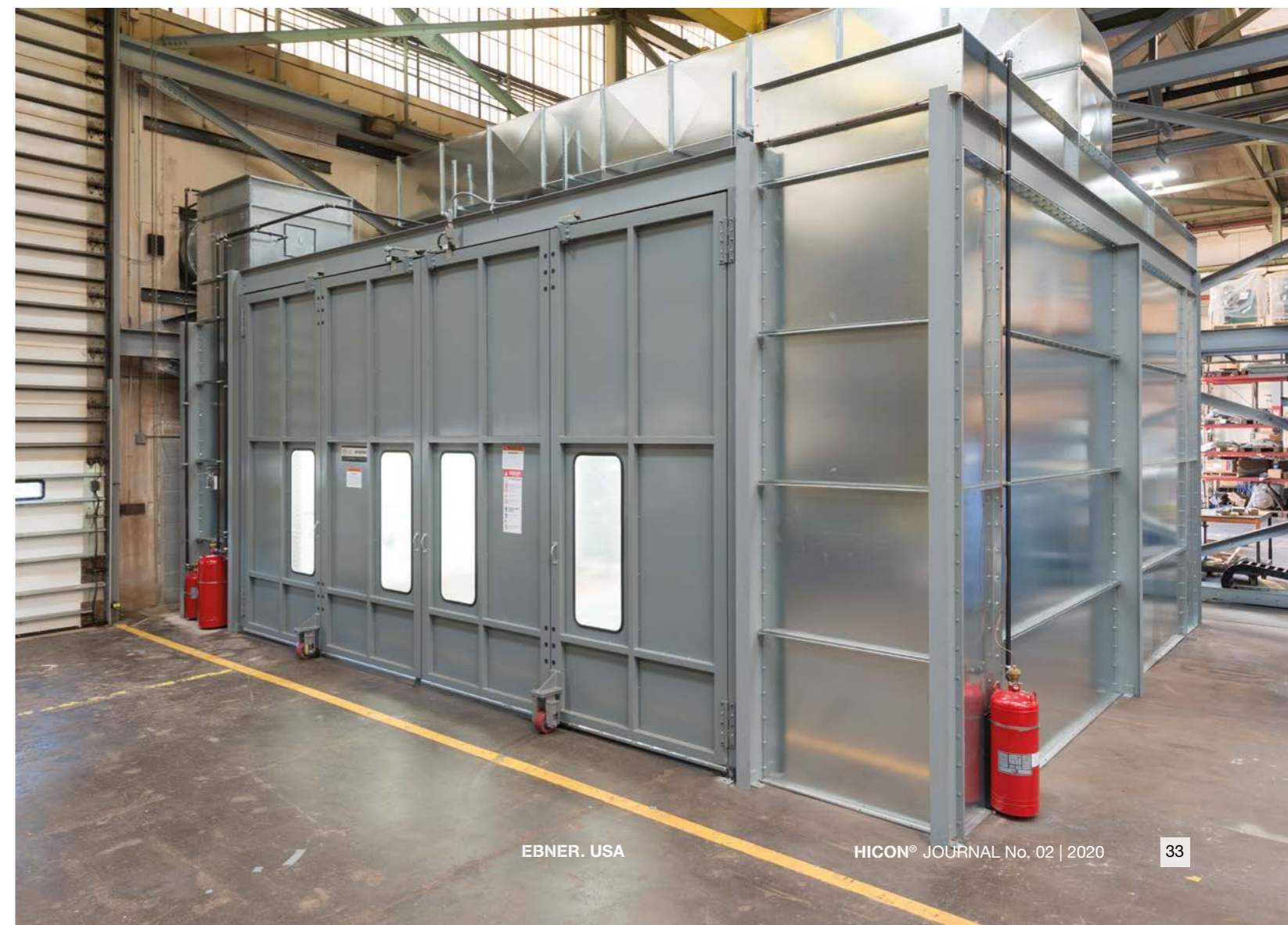
Paint booth in the workshop at EBNER USA
