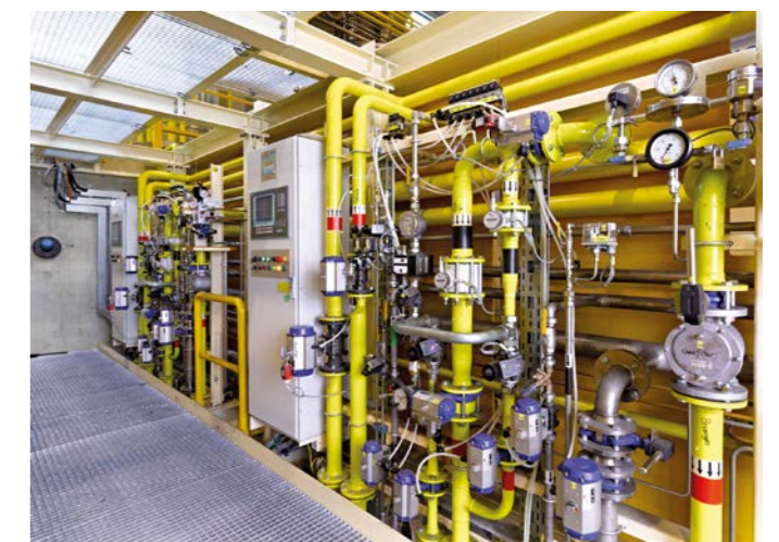
2 valve stands and the associated control cabinets
