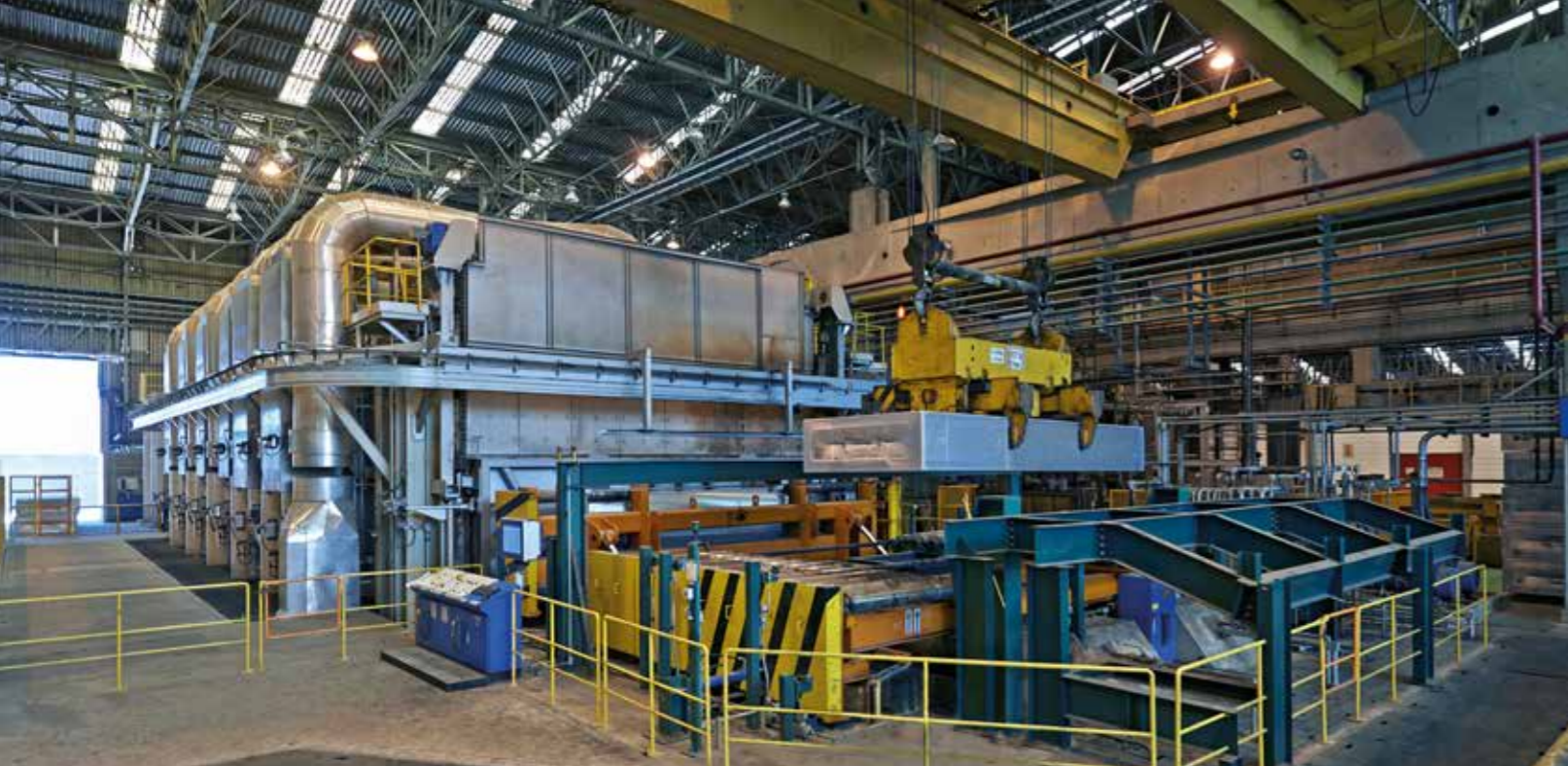
EBNER pusher furnace facility in Brazil
