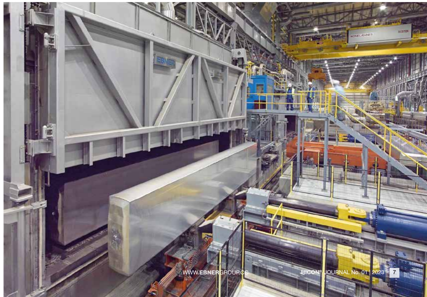
EBNER pusher furnace (furnace entry) with an extremely long rolling ingot in a state-of-the-art plant
