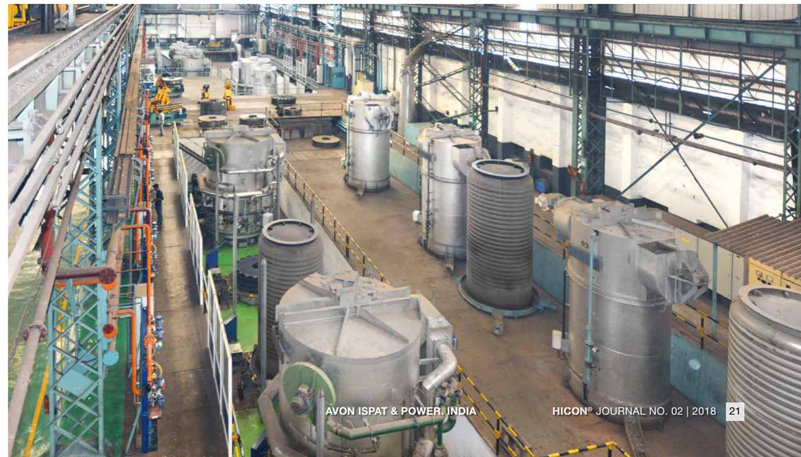
Several expansion phases of EBNER furnaces
