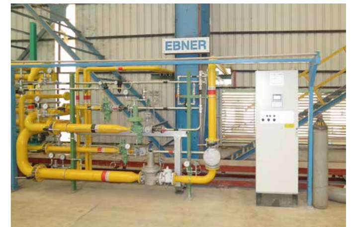
Gas engineering by EBNER
